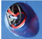
The ESC is located inside the forward vent hole, just aft of the cowling's anti-scuff plate.
